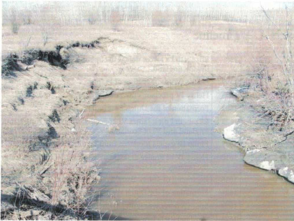
Photo # 17. Looking NE off bridge on Trans-Canada Trail at erosion on S-facing bank of Tawatinaw River at location TW13 on April 21, 2011
