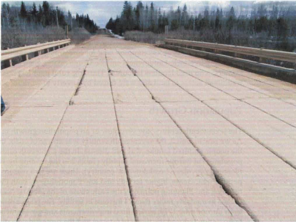
Photo # 9. Looking E at severely eroding cement bridge deck at location TW01 NW of Perryvale on April 21, 2011
