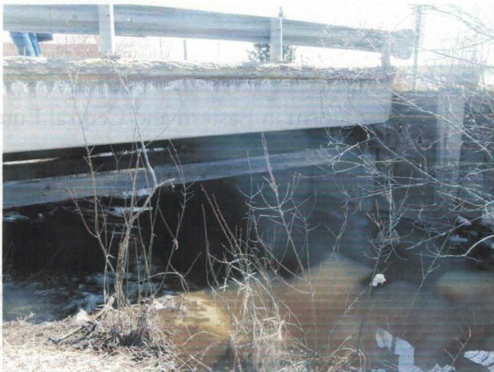
Photo # 13. Looking SE at degrading cement bridge deck at location TW05 in the village of Tawatinaw on April 21, 2011
