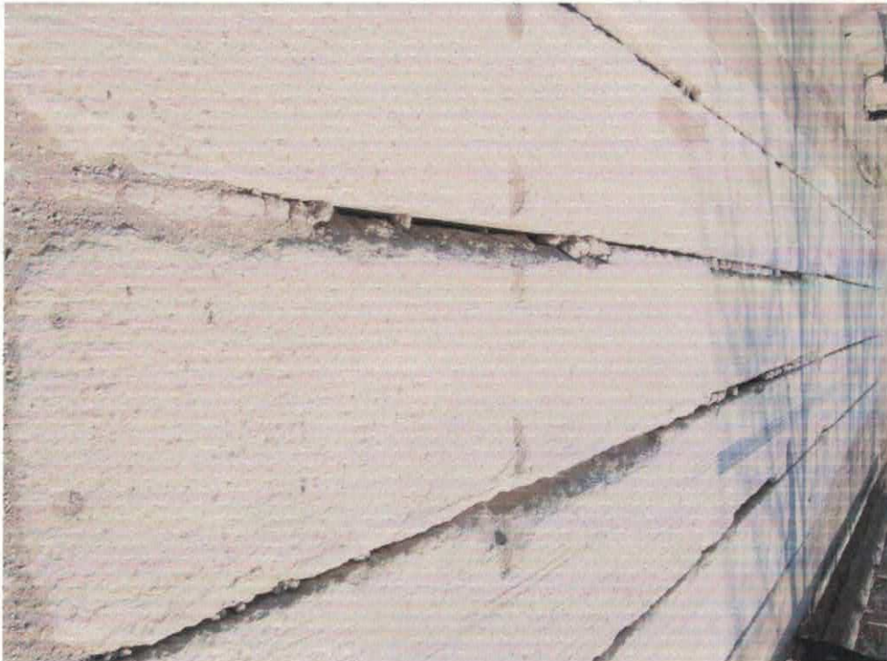
Photo # 16. Looking S-SE at heavily degrading cement bridge deck at location TW12 on April 21, 2011
