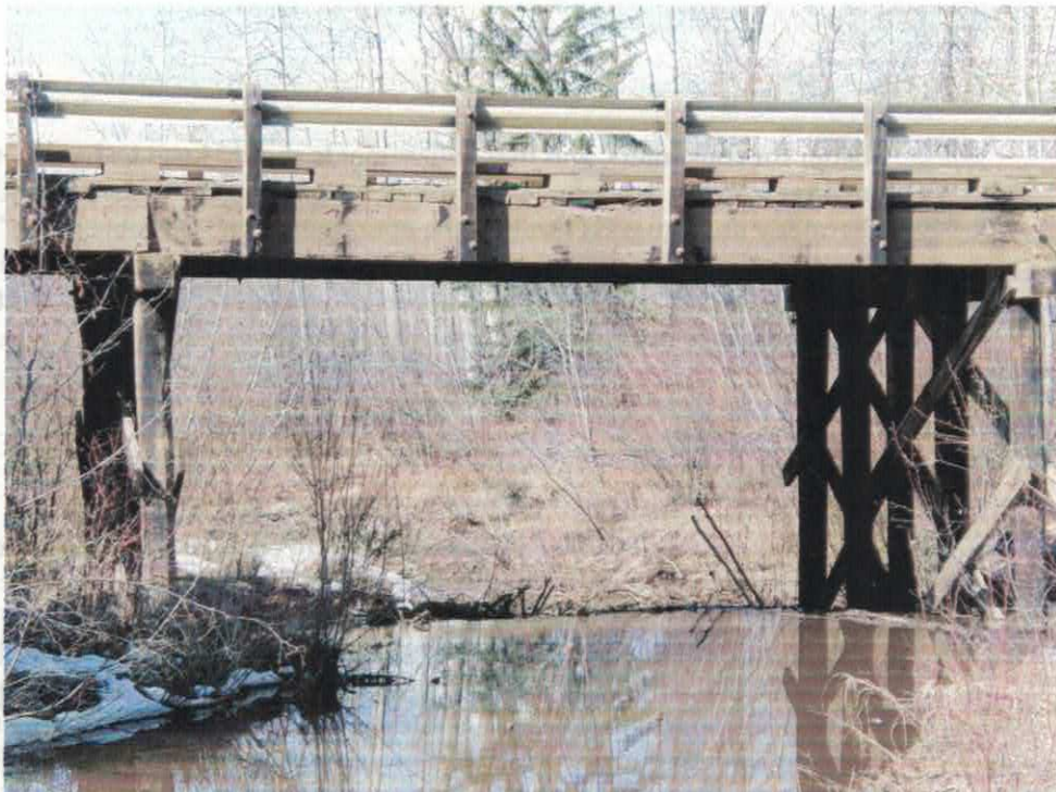
Photo # 3. Looking E at eroding wooden bridge and beaver dam constructed beneath bridge at location TW10 (conjunction point of Little Pine and Colinton Creek) on April 21, 2011
