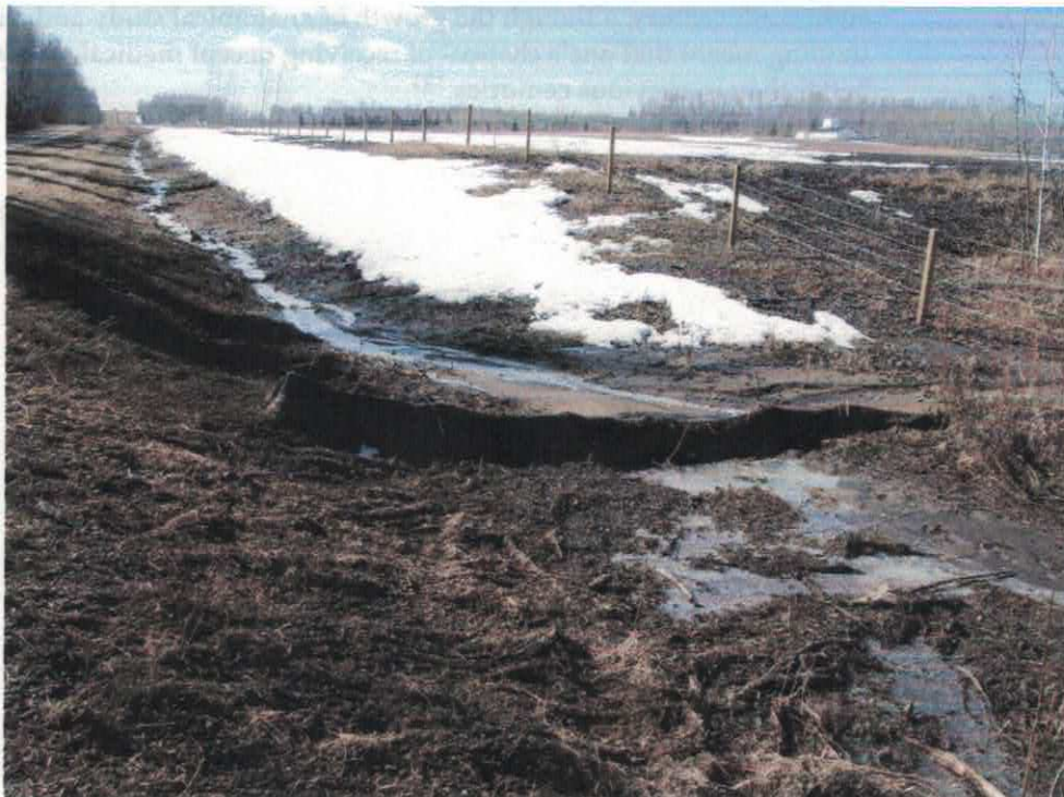
Photo # 2. Looking S at inadequate silt fencing installation at location LP1B 1 on April 21, 2011
